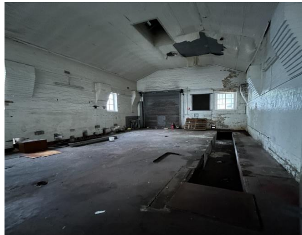
Figure 16 – Interior of the substation facing northeast.
